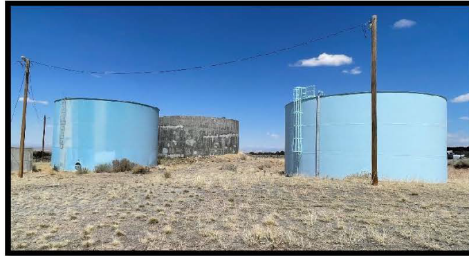
Figure 10-1 Oak City Water Storage Tanks
